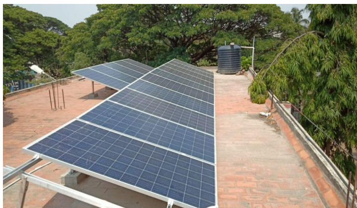
Figure 6 Solar System for Electricity in Private Bungalow (Dharmaj)
